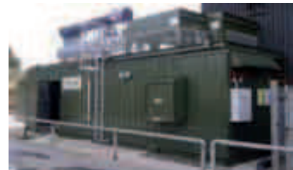
Fully containerised 1200kWe CHP Unit, including full heat recovery, being supplied to Queen's University Belfast
